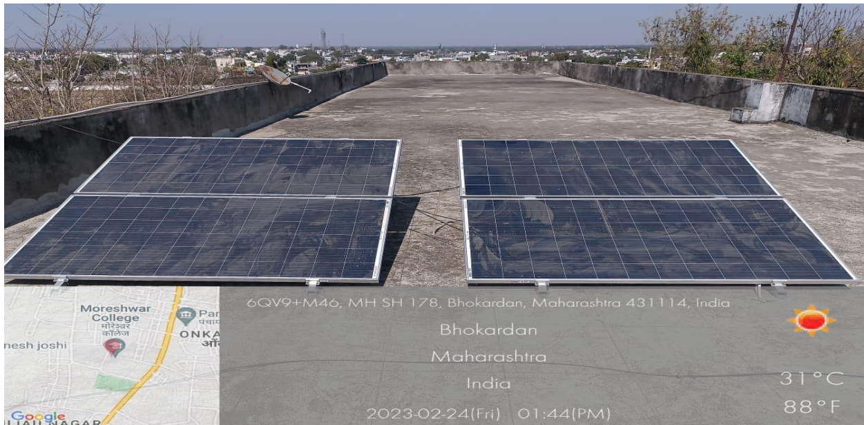
SOLAR SYSTEM PANNELS
